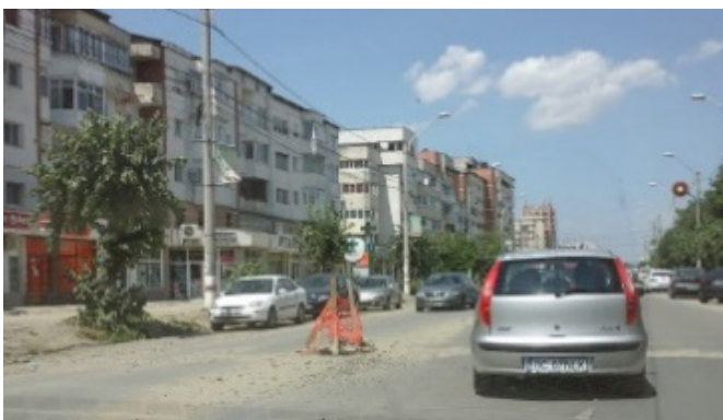
Figure 3.50: Construction with no protection or segregation of work zone and general traffic—Romania.
