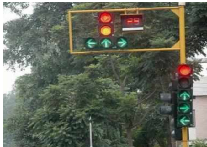
Figure 6.17: Traffic control signal for vehicles in India.
