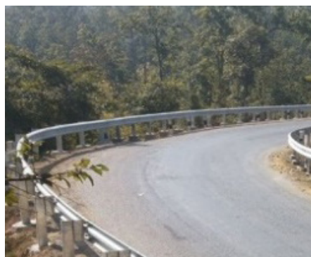
Figure 5.36: Semi-rigid barrier on horizontal curve in Nepal.
