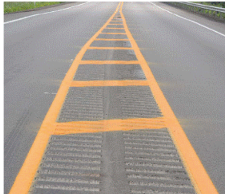
Figure 5.97: Flush median with rumble strips.
