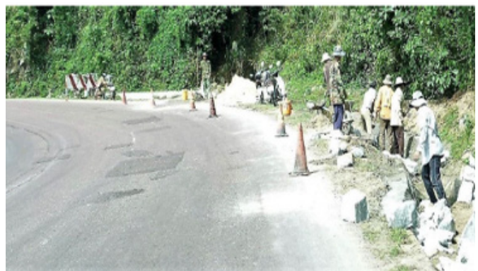
Figure 3.51: Complete lack of roadworker protective clothing or adequate workzone demarcation.
