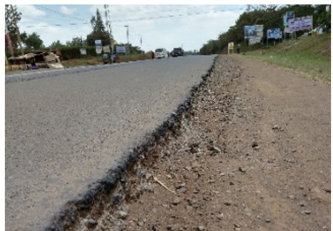
Figure 5.10: Pavement edge drop.
