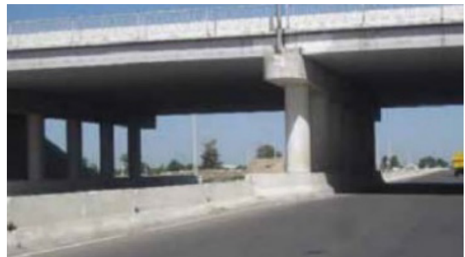
Figure 5.77: Shielded piers with rigid barriers. An appropriate end treatment (cushions/impact attenuators) should also be applied on barrier systems.
