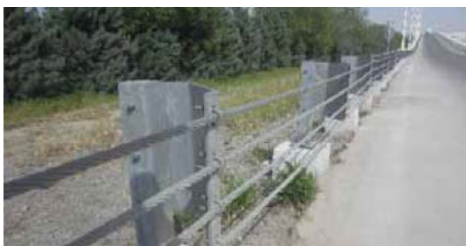
Figure 5.83: Flexible barriers with too large posts.
