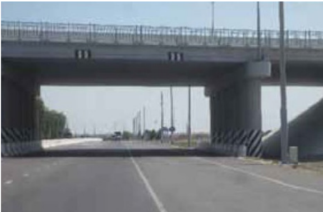
Figure 5.68: Unshielded overpass piers.
