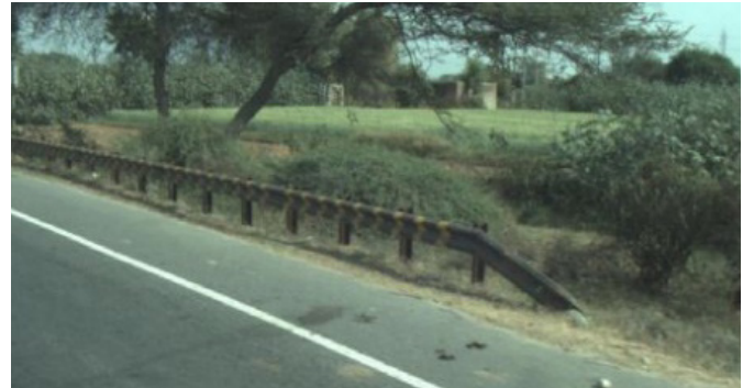
Figure 5.88: Unsafe ramped end of semi-rigid barrier that can launch an impacting vehicle.
