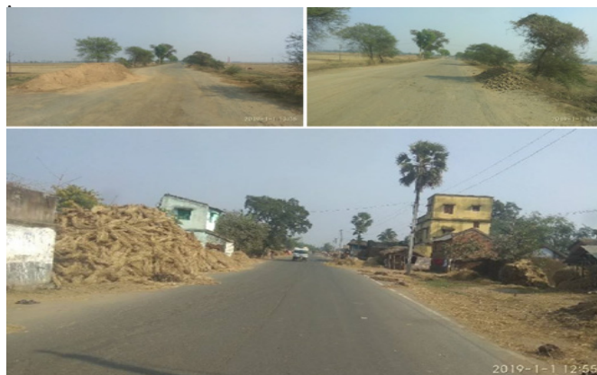
Figure 3.53: Stacked construction material unprotected or contained along the highway—India
