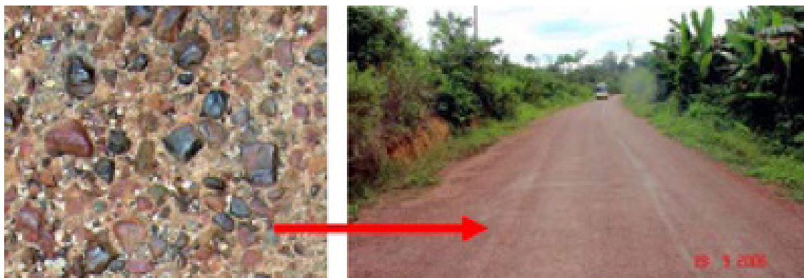
Figure 5.122: Otta seal surfacing on low volume road in good condition with satisfactory results. (left image: close-up of the otta seal surfacing).
