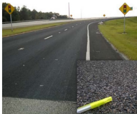
Figure 5.123: High friction surface treatment on high-risk curve.
