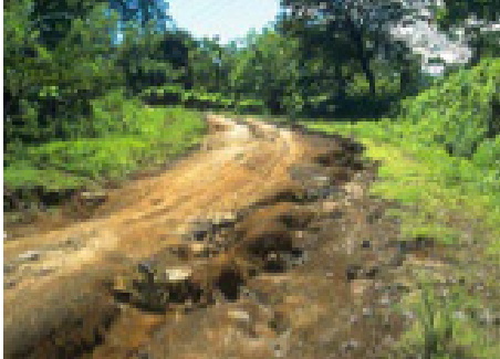
Figure 5.135: Poorly drained road with rough driving surface (sediment source).
