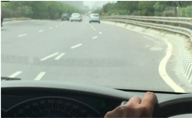
Figure 5.165: Unexpected deviation of line marking—India
