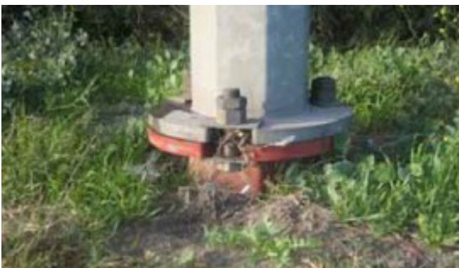
Figure 5.169: Slip-base lighting column suitable for high-speed roads with little pedestrian activity and parking.
