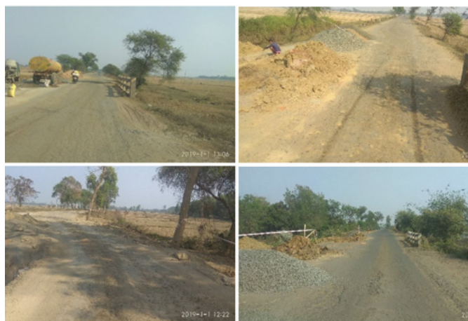
Figure 3.52: Unprotected work areas and materials—India
