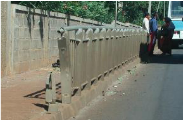
Figure 4.10: Poorly maintained pedestrian guardrail—Maintenance Inspection.
