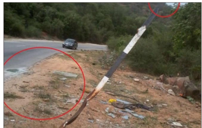
Figure 5.50: Broken signs without maintenance in India.
