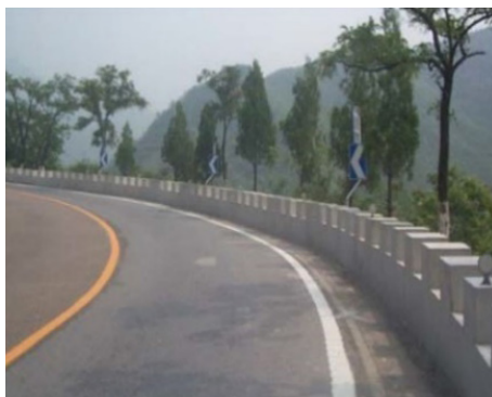
Figure 5.35: Concrete barrier on curve section with chevron alignment signs.
