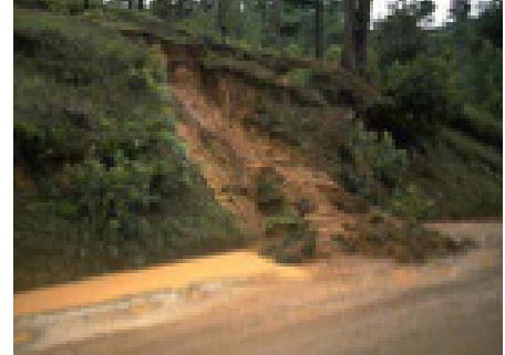
Figure 5.137: Slide material blocking drainage ditches.
