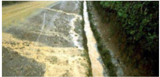
Figure 5.143: Armor ditches with vegetation, rock, masonry, or concrete to resist ditch erosion.
