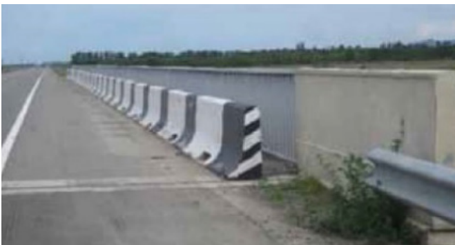
Figure 5.89: Unsafe gap between guardrail and concrete
