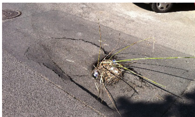
Figure 3.54: Poorly maintained road surface—Romania.
