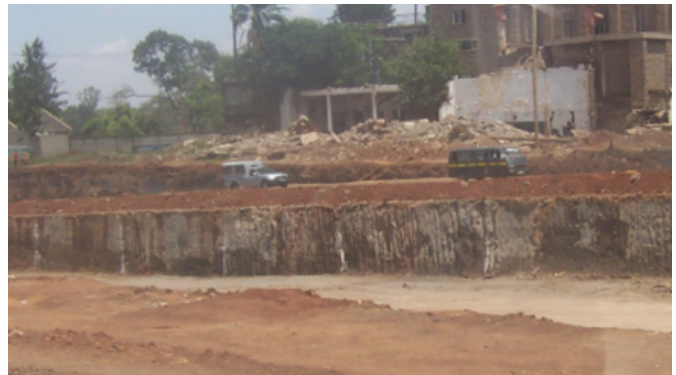
Figure 3.49: Major excavation with no protection or segregation of work zone and general traffic—Kenya.
