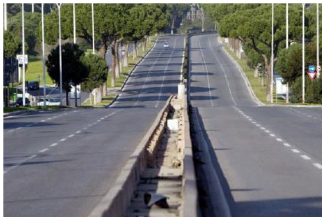
Figure 5.149: Hazardous vertical curbs on high-speed road.
