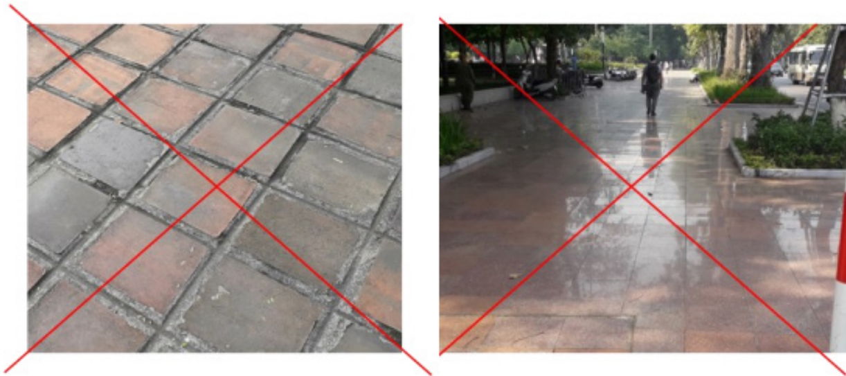
Figure 4.2: No tripping hazards or slipper floors.
