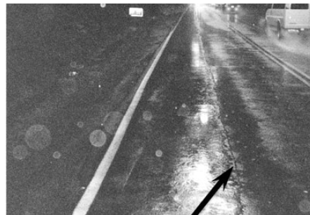
Figure 5.131: Edge of partial pavement overlay causing water to be retained on surface
