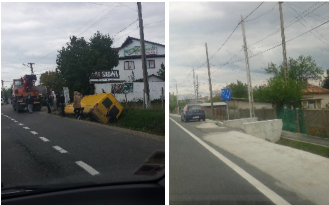
Figure 5.66: Uncovered drain and unsafe culvert—Romania.
