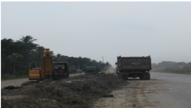
Figure 3.48: Construction work going on without any temporary safety measures—West Bengal.
