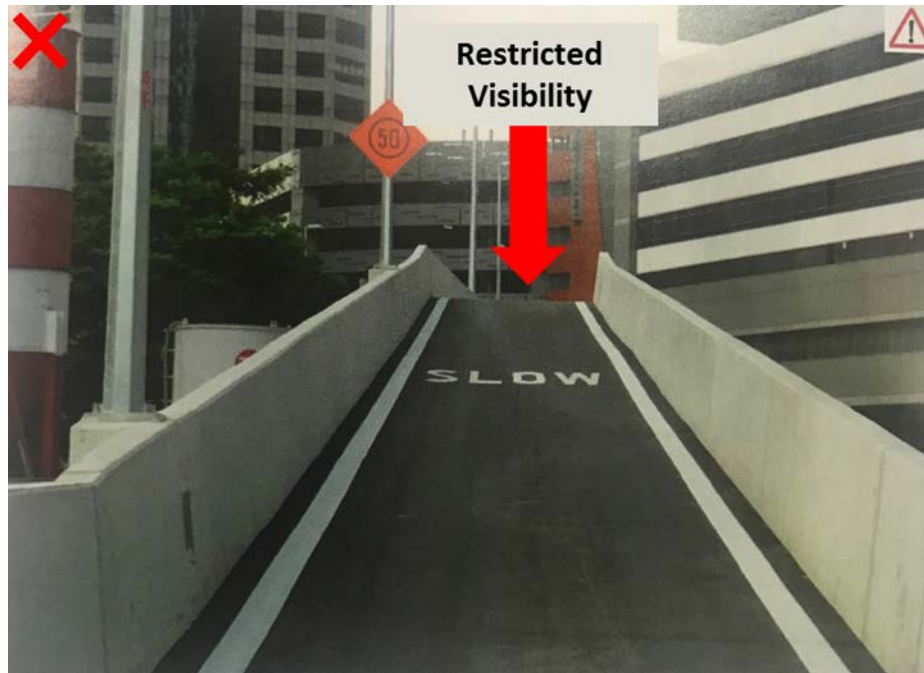
Photo 5.3. Inadequate Visibility Along Vertical Curve, Singapore
