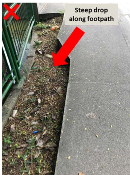
Photo 5.6. Hazardous Footpath, Singapore
