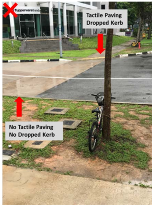
Photo 5.5. Inadequate Crossing, Singapore
