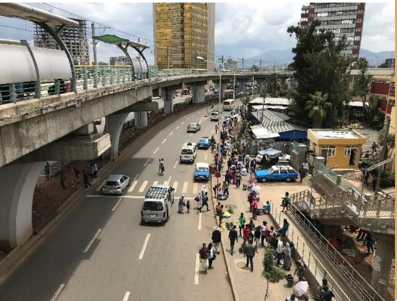
Problems in sidewalks identified along LRT corridors
