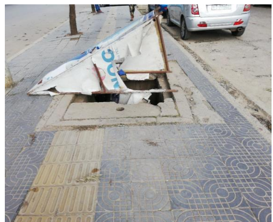
Pedestrian traffic obstacles
