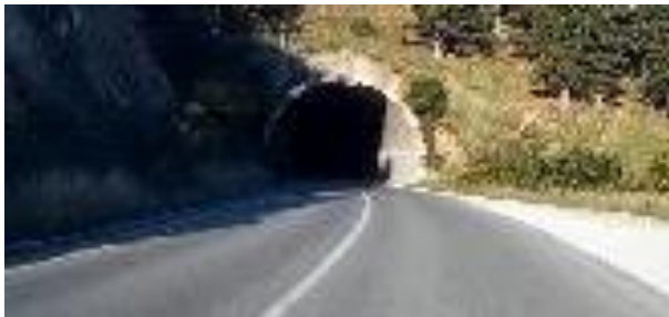
No lights in tunnel
