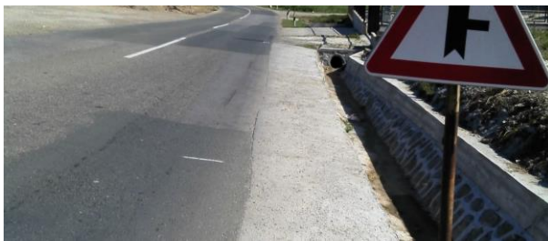
Unsafe drainage system, with headwall
