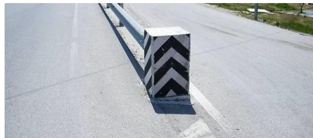
Dangerous “end treatment”- concrete block
