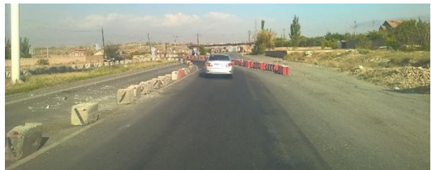
Dangerous work zone
