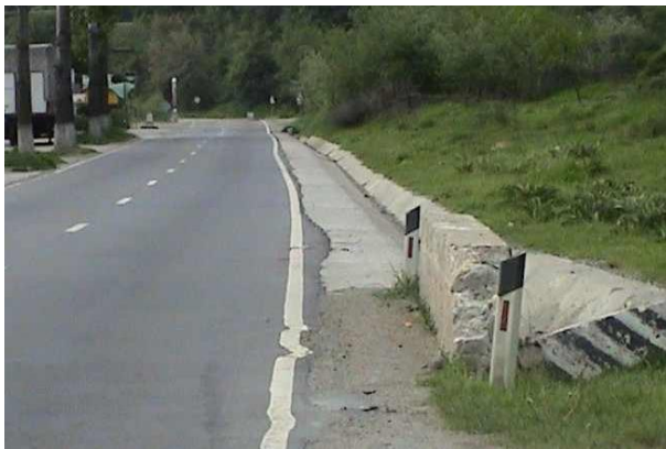
Unsafe headwall of a culvert
