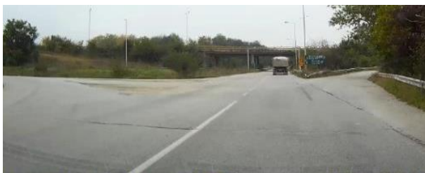
Missing channelisation in junction
