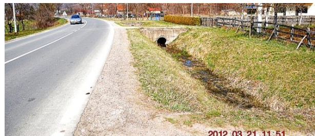
Unsafe drainage system, U-Type with headwall
