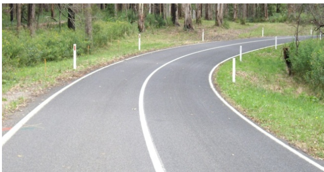
Guide posts and linemarking. Source: ARRB Group.
