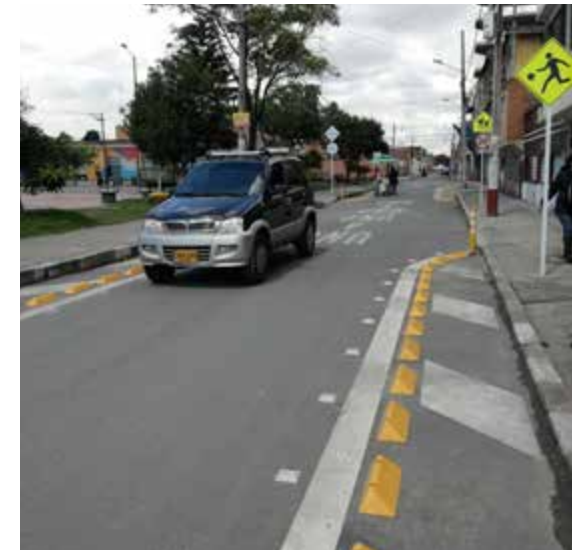
Figure 10.10 | Medium-Term Materials Installed in Tunjuelito to Form a Choker after Success of the Temporary Pilot Project
